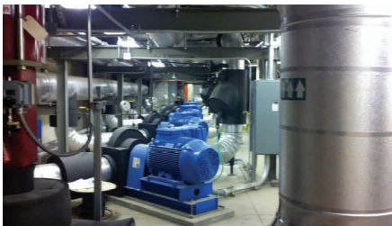
Chilled Water Storage
